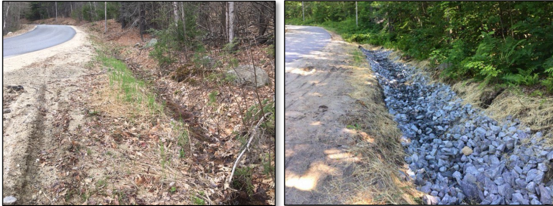
Eroding ditch on Staples Hill Road was reshaped and armored with rock, road shoulder reshaped and bare areas mulched.
