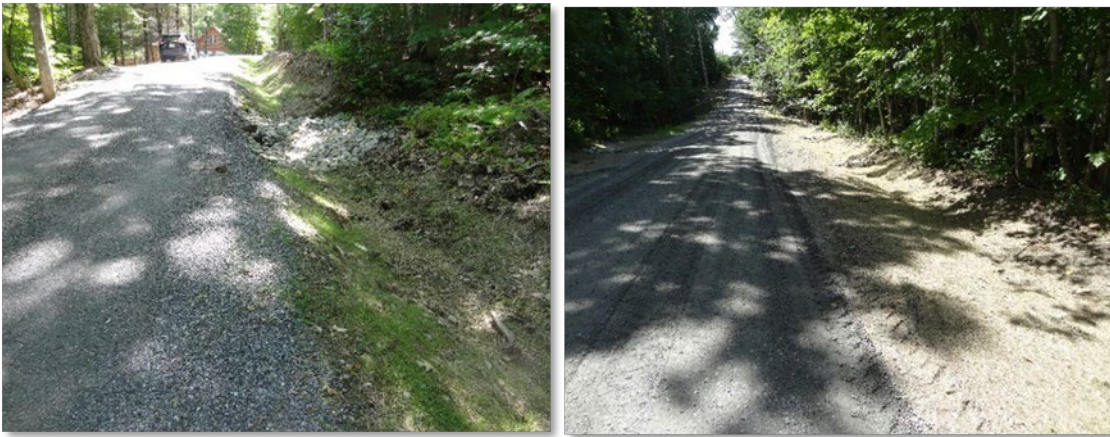
Typical dirt road BMPs at the Bacon Road site in Mercer.
