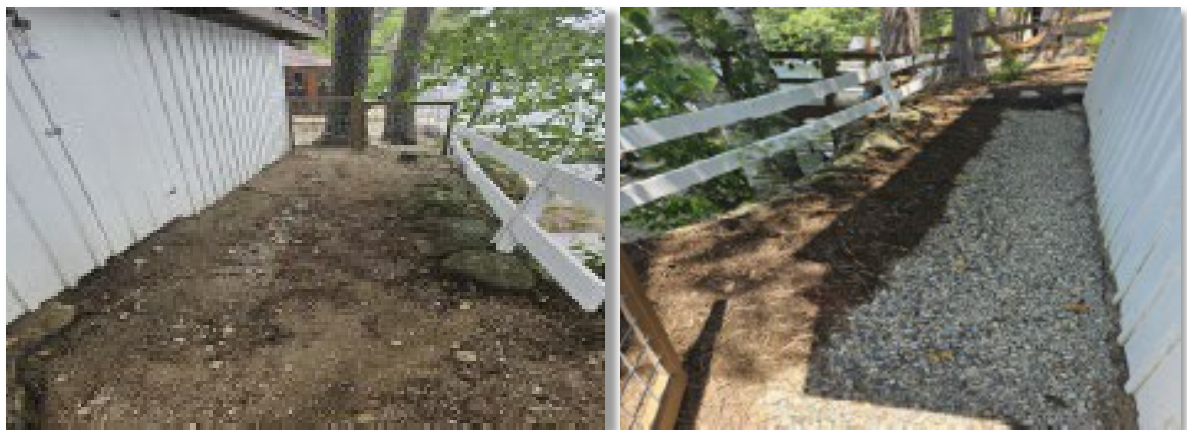
Infiltration trench constructed by the Acton-Shapleigh Youth Conservation Corps in 2023 on Mousam Lake. The left side shows the “before” condition, and the right side shows the “after”.
